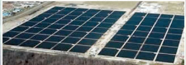
Sarnia Photovoltaic Power Plant
